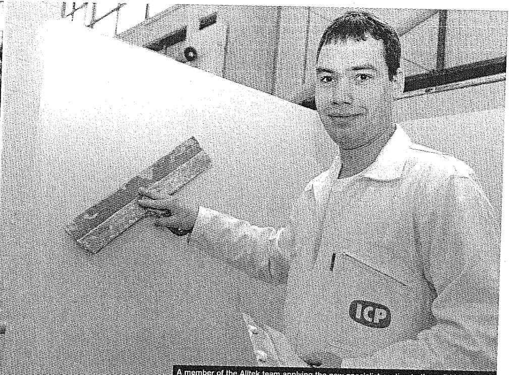
A member of the Alltek team applying the new specialist coating to the solid block wall.
